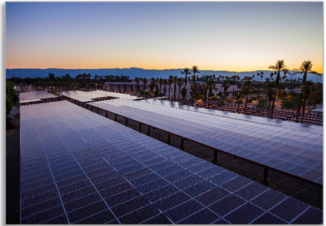
Solar Photovoltaic System
